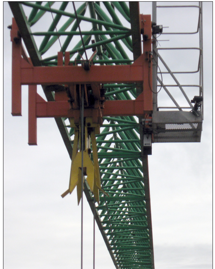
Orlaco Quick Fit Set with Battery pack and Camera AFZ, Orlaco Autocontact and the Orlaco Spectrum Scanner mounted on the trolley of a tower crane.
